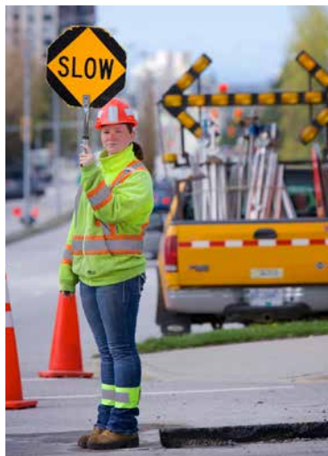
Use a variety of devices in your work zone to alert drivers to your presence. Cones alone are not enough.
